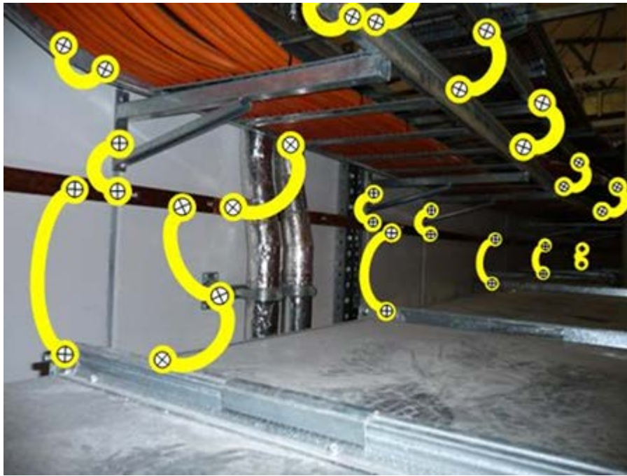
Figure 8-5 Examples of bonding natural metalwork, on an existing synchrotron, #2.
