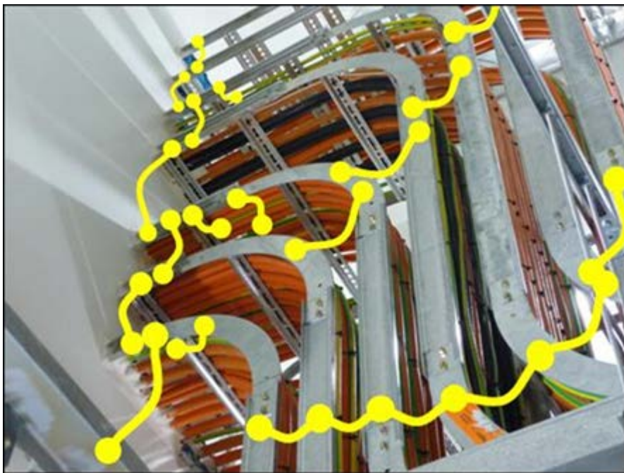
Figure 8-6 Examples of bonding natural metalwork, on an existing synchrotron, #3.
